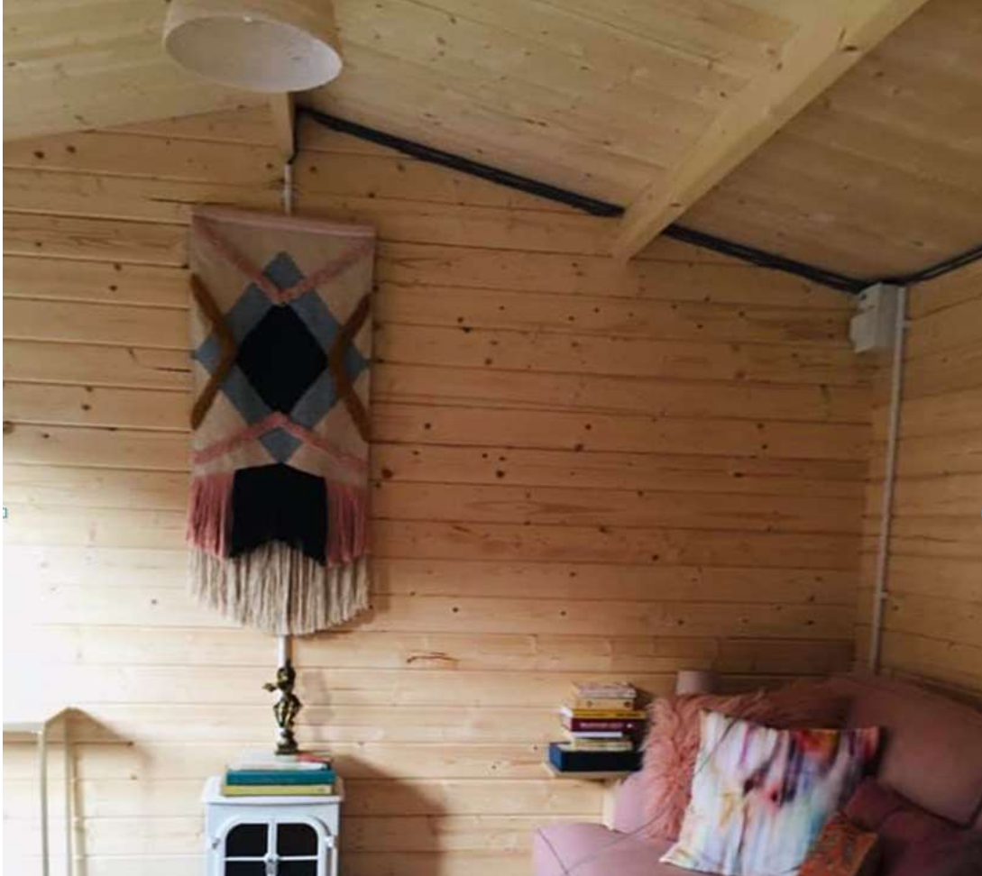
This image above shows the internal cabling and the white conduit which will be visible within the completed building.
